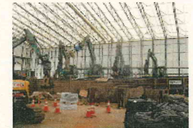
Soil reception / separation facility of Interim Storage Facility (Okuma Town)
